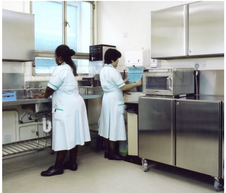
GEC Anderson stainless steel kitchen.
