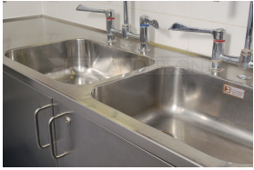
Integrated sinks within stainless steel worktop, mounted on stainless steel base cabinets.
