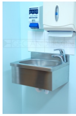
Ward kitchen - sinktop, cabinets and drawers. Wall hung WB45 basin.
