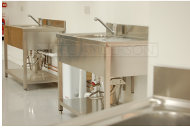
Decimetric sink and drainer with legs and frame and V55 Gypsum Separator
