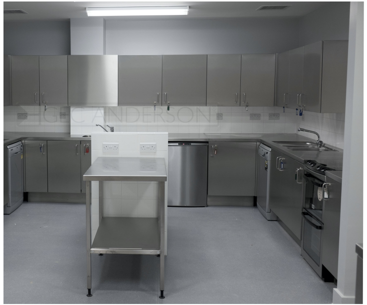
Stainless steel wall cabinets, over worktops with base cabinets.
