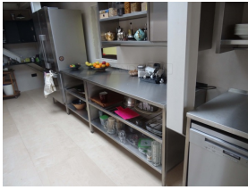
Stainless steel counters with supports and undershelves.
