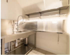
Pre-rinse sink and shelving.
